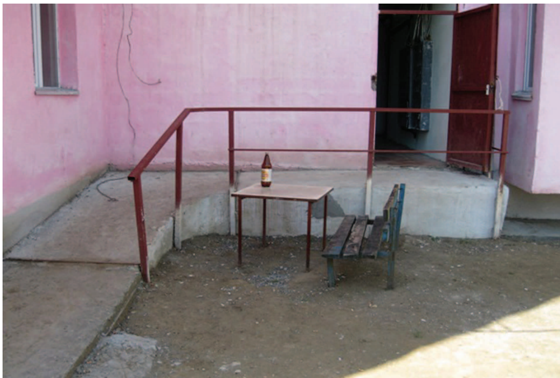
Ramp for the Persons with Disabilities at the entrance of the Tskaltubo accommodation.
