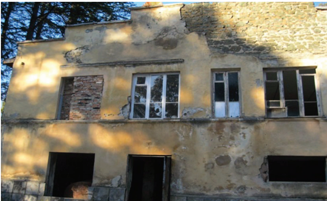
The “Ushishroeba” sanatorium building in Tskaltubo from which the IDPs were transferred.
