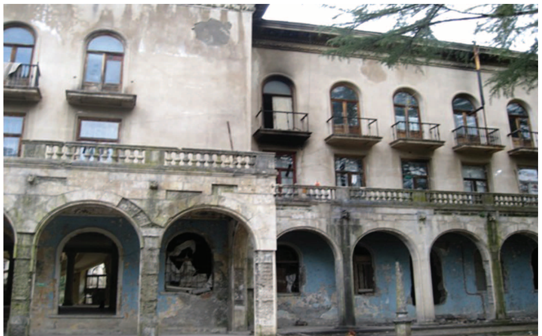
Tskaltubo "Sanatorium Imereti". The building is wrecked. Transfer of IDPs had not occurred.
